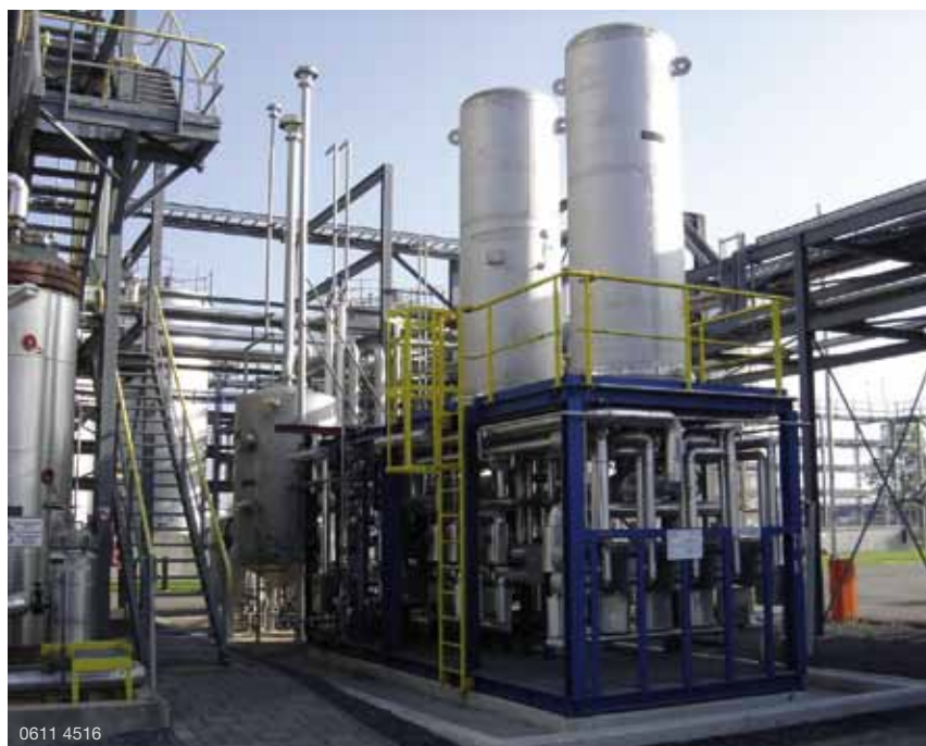
0611 4516 Skid mounted PERVAP™ membrane plant
